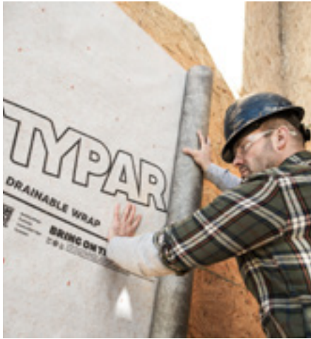
Figure 3. The American Architectural Manufacturers Association defines WRBs as a surface or a wall responsible for preventing air and water infiltration to the building interior.
