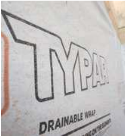
Figure 2. Building wraps made of polyethylene or polypropylene fabric have been a popular method of protecting homes and buildings against moisture intrusion since the 1970s.
