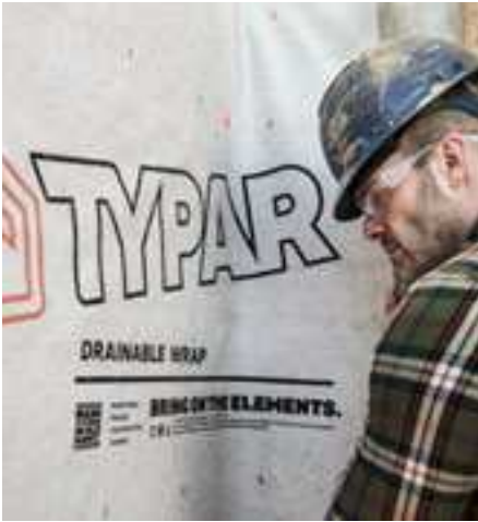
Figure 4. As building assemblies have gotten tighter, building wraps have taken on a new function—helping to remove trapped water from the building enclosure.
